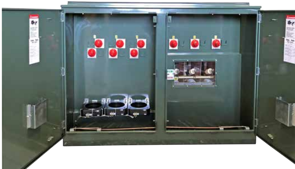
Rear view of the 25kV padmount design (Breaker terminals on the left with CTs. An AutoJet switch on the right.)
