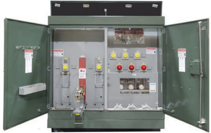
Figure 2 - Phase 2 (nominal B Phase) fuse panel in Compartment 4 is shown in the open position, with hinged roof open.
