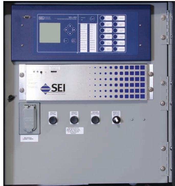
Figure 4 - SEL-451 Relay, with SEI UPS.
