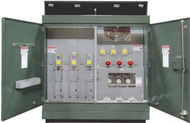
Figure 1 - Fuse Compartment 4 (left) and Switch Compartment 3 (right), shown with hinged roof open.
