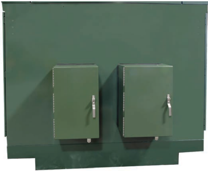
Figure 3 - Side view showing dead-front to live-front base adapter (bottom) and the two back-to-back switch motor operators on the side.
